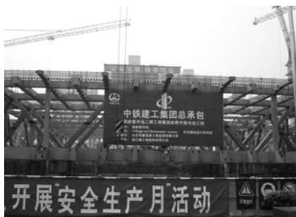
The construction site of NLC's new eight-story digital library — a massive and modern design by German architects Engel und Zimmermann — shows girders swinging through the air and signs identifying the construction company and exhorting safety.
